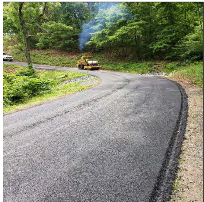
The Sanitary District staff works to widen the roadways and shoulders on the trails within Shawneeland. The staff work diligently to make the roads safer for residents and emergency personnel.
