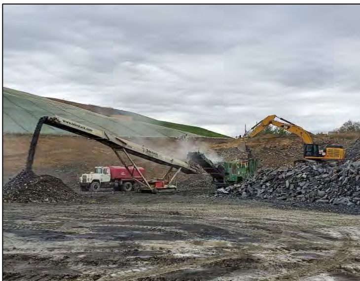
Contractor is nearing completion of the rough grading of MSW Cell 3A. This photo shows blasted rock being processed into useable material.
