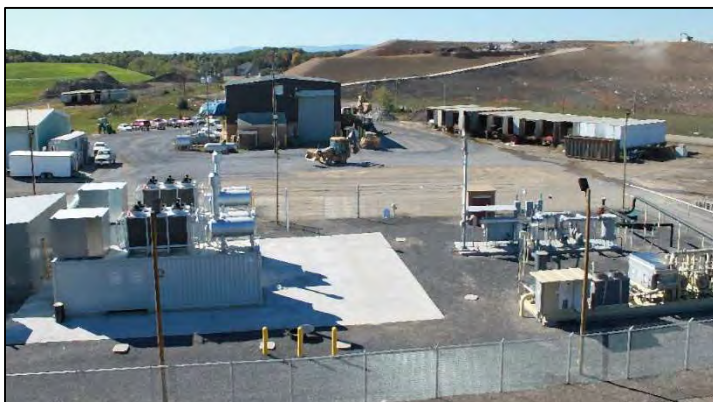
Landfill Gas to Energy Plant
