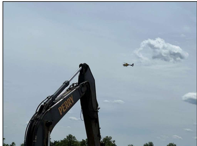
An air ambulance helicopter circles to land at the airport with an excavator boom shown in the foreground. The airport is experiencing an immense period of growth through capital projects while maintaining operations.
