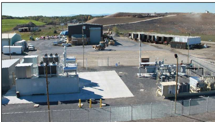
Landfill Gas to Energy Plant
