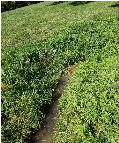
Leak emerging from the ground
