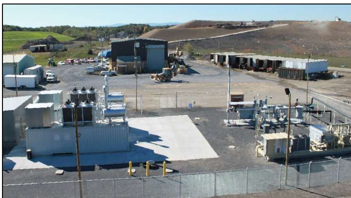
Landfill Gas to Energy Plant
