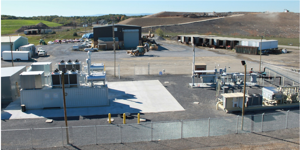
Landfill Gas to Energy Plant
